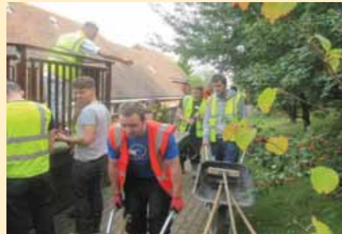
Our trainees, in their annual charity event, completely renovated a one acre garden at Delmelza House Hospice. The value of the trainees' time, material and the hire of heavy machinery was £28,000.
