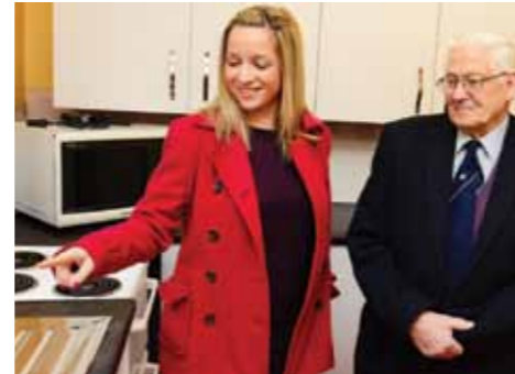
We re-fitted the church hall kitchen for local people who use it as valuable community meeting point
