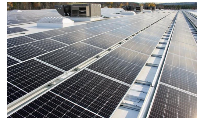
Figure 2 - Monocrystalline PV installation on flat roof
