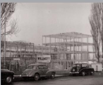
Letchworth College of Technology 1957 See Spirella Building on right behind the trees
