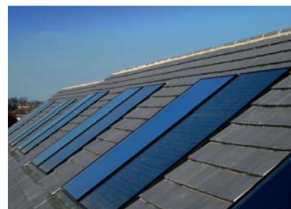
Micro-generation solar panels
